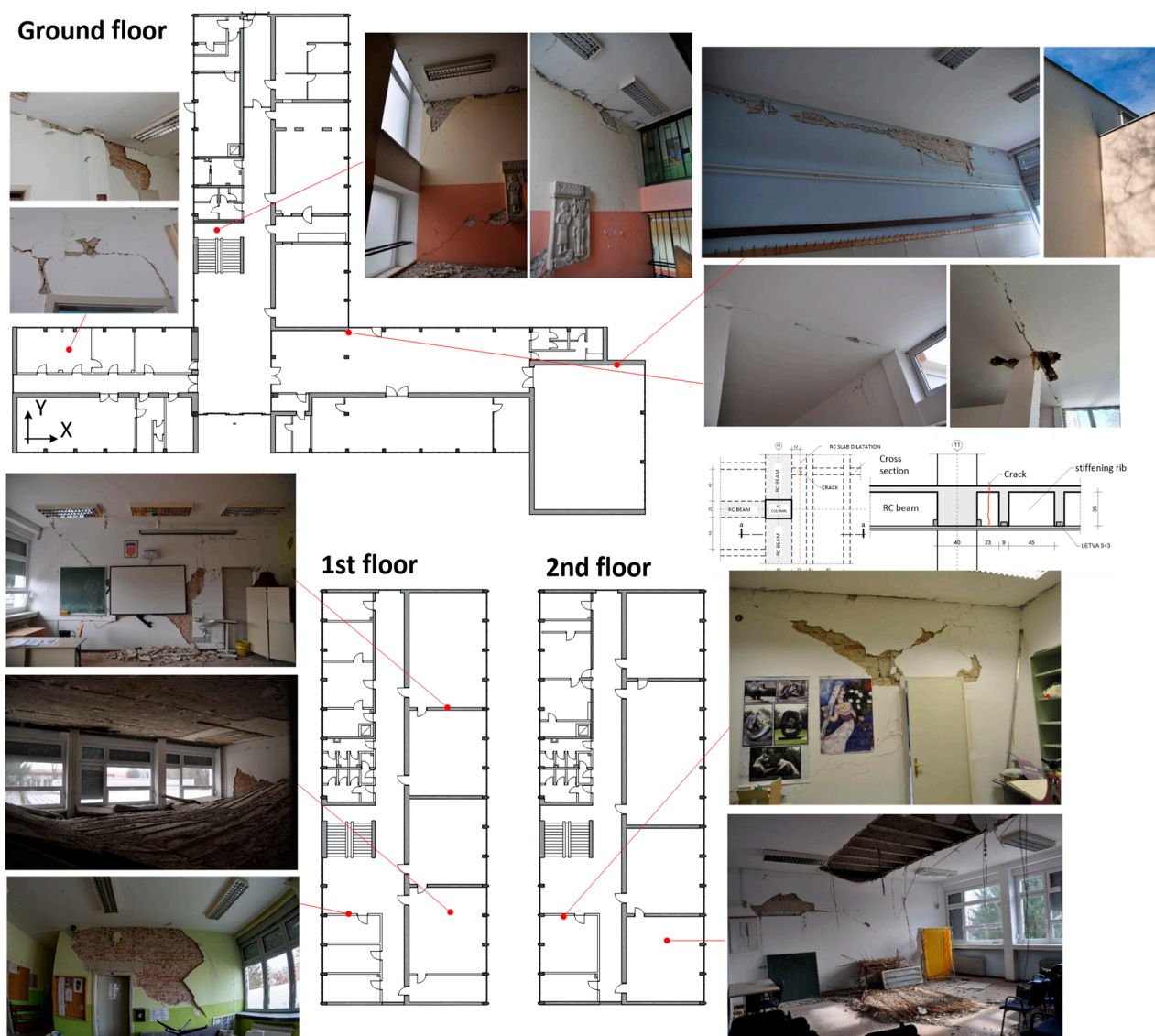
Figure 6. Photographs of damage to the building (photos: courtesy of Joško Krolo and Karlo Jandrić, 2021; and CCEE, 2021).
