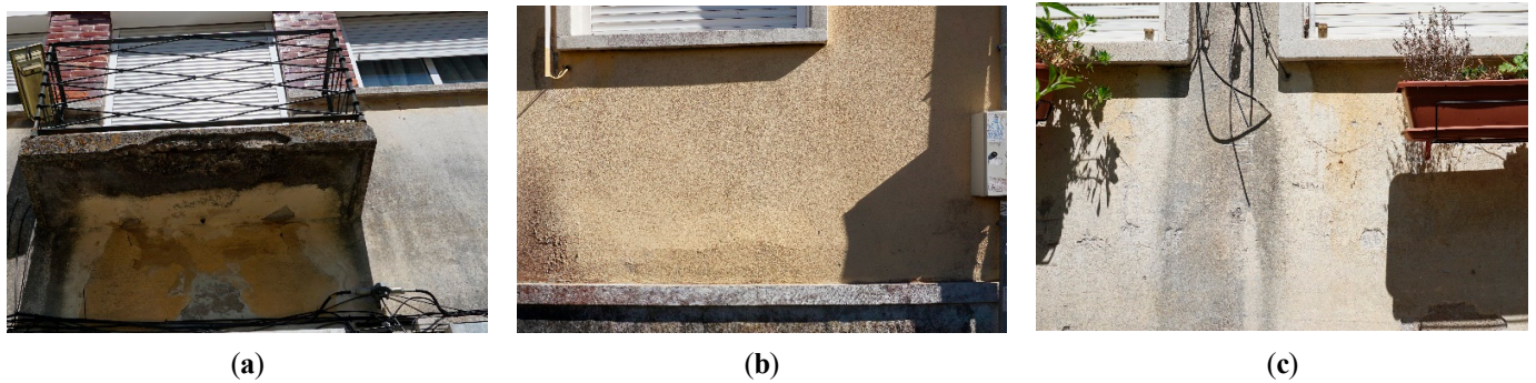
Figure 4. Different types of loss of adhesion: detachment (a), bulging (b) and crumbling/spalling (c).
