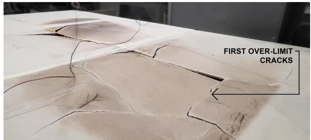
Figure 11. The condition of the structure at the end of the test.
