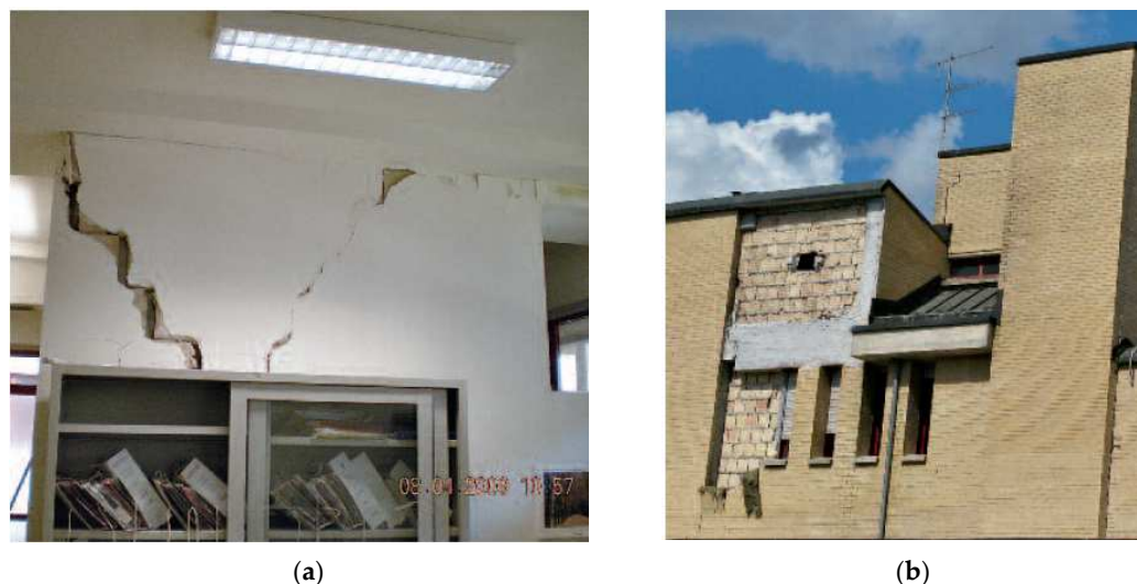
Figure 1. Examples of nonstructural damage detected in the San Salvatore hospital in L'Aquila after the 2009 event (pictures from [7]): (a) damage to internal partitions; (b) collapse of masonry veneers outside one of the hospital buildings.
