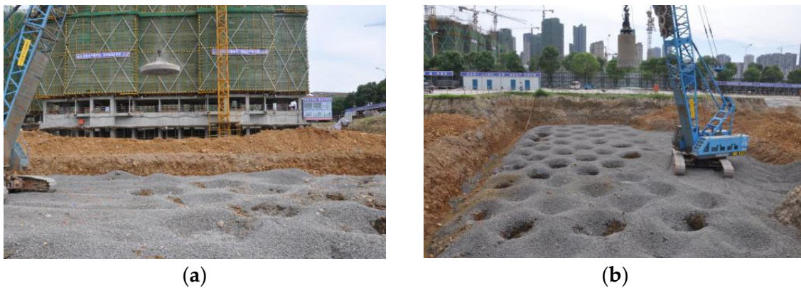
Figure 4. Construction photo of combined hammer: (a) flat hammer; and (b) column hammer.
