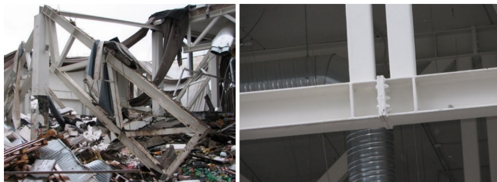
Figure 1. Deadly store roof collapse due to the failure of the metal joint.
