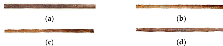
Figure 9. Corroded steel bars after rust removal: (a) cross-sectional loss = 10%; (b) cross-sectional loss = 20%; (c) cross-sectional loss = 30%; (d) cross-sectional loss = 40%.
