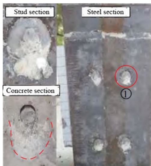
Figure 11. Photo of stud shear failure.
