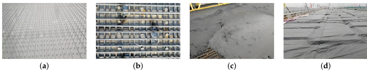
Figure 6. UHPC construction process: (a) Welded shear stud; (b) Steel mesh; (c) Pouring UHPC; (d) Steam curing.
