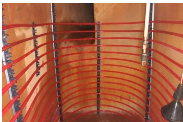
Figure 1. Heat exchange circuit installed in the cistern of the Apolonio Morales 29 office building.
