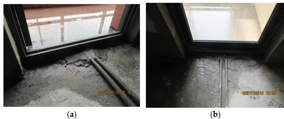
Figure 4. Leakage problems in the water storage tests. (a) Leakage at the small balcony anti-seepage; (b) leakage at the kitchen threshold seepage.
