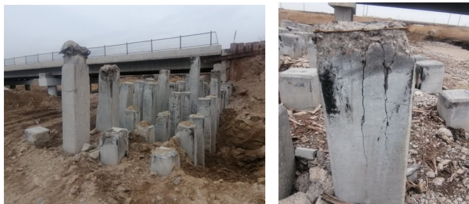
Figure 1. Undriven piles of the bridge under construction over the Shu River (Zhambyl Region, Republic of Kazakhstan).
