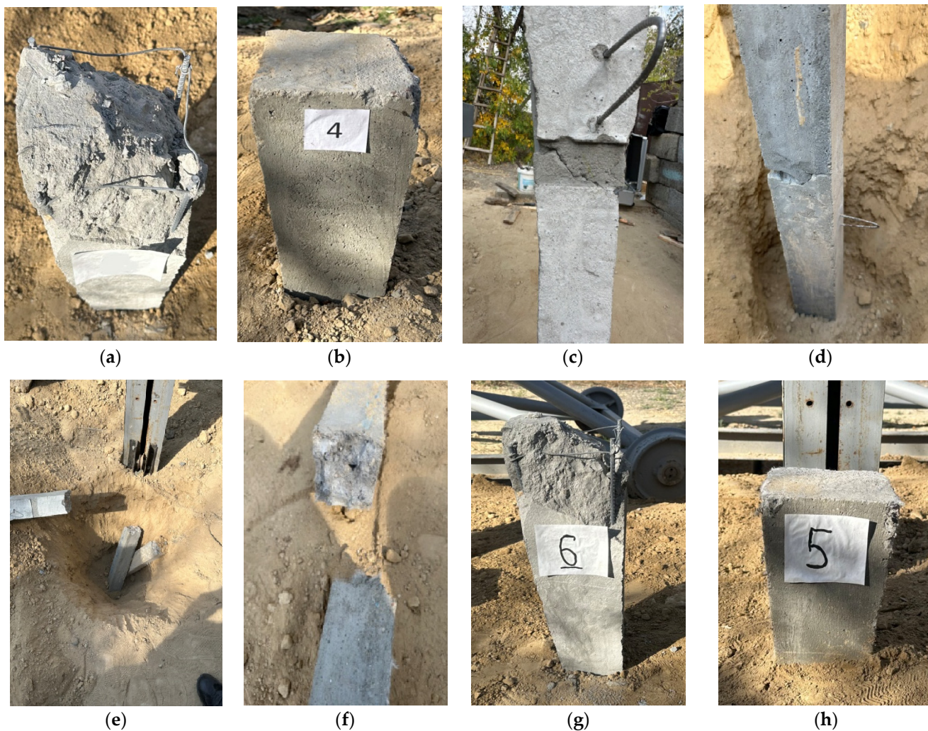
Figure 9. Driven piles and their defects: (a) SFC-1; (b) PFC-1; (c) SFC-2; (d) PFC-2; (e) SFC-3; (f) PFC-3; (g) SFC-4; (h) PFC-4.
