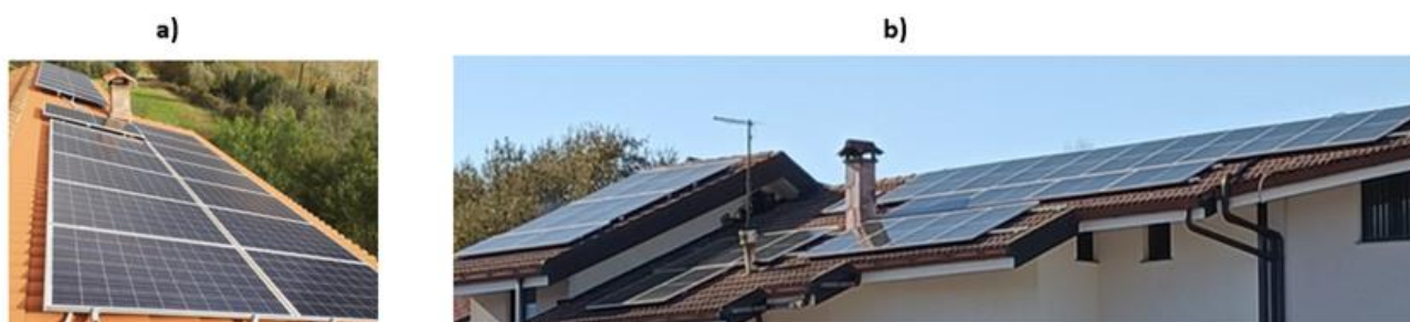
Figure 1. (a) Green Family photovoltaic system, (b) Smart Worker and Young Family photovoltaic system.
