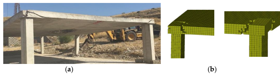
Figure 19. Cracks close to the end of the second central column removal: (a) actual structure and (b) model using LS-DYNA.
