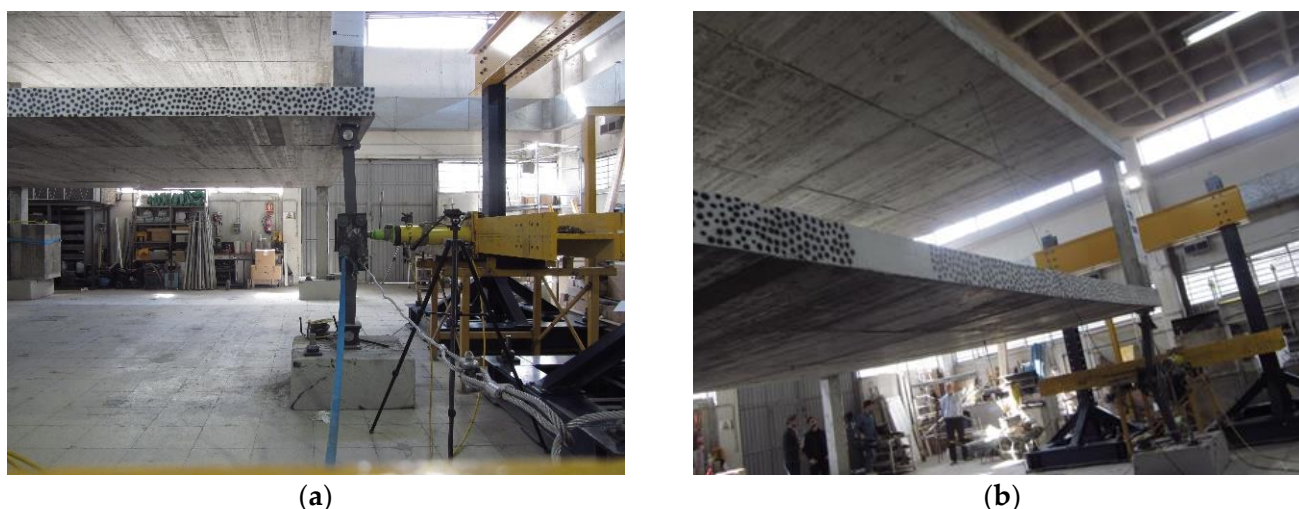
Figure 1. (a) View of the steel column with slight rotations outwards before deblocking of the central hinge. Cables used to deblock the hinge are visible in the foreground. (b) View of the structure after the sudden removal of the vertical support at the location of the steel column.
