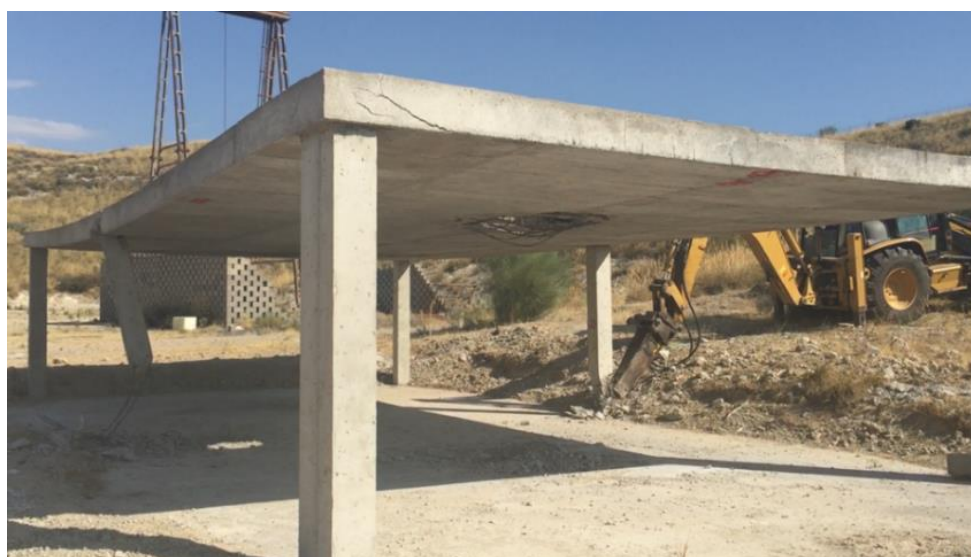
Figure 17. Cracks after one of the central supports was demolished.
