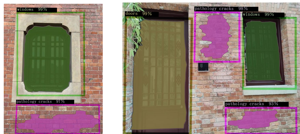
Figure 11. Based on Mask R-CNN crack area detection model, the James Jackson Gymnasium area detection results of pathology cracks are displayed. Green is marked as window class, yellow is marked as category, and purple is marked as architectural heritage pathology cracks.
