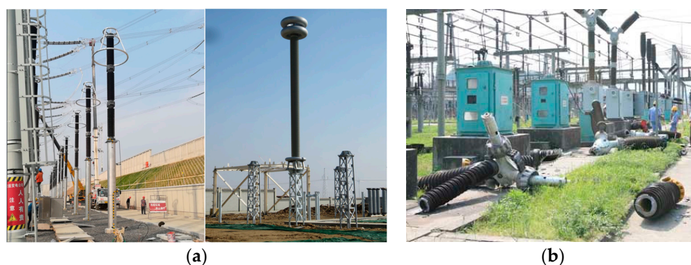
Figure 1. Example of seismic fragile pole-type equipment in engineering (photo by the author) and damage of an electrical substation within the Sichuan electric power grid during the 2008 Wenchuan earthquake (cited from [25]). (a) Pole-type cylindrical equipment; (b) Earthquake damage.
