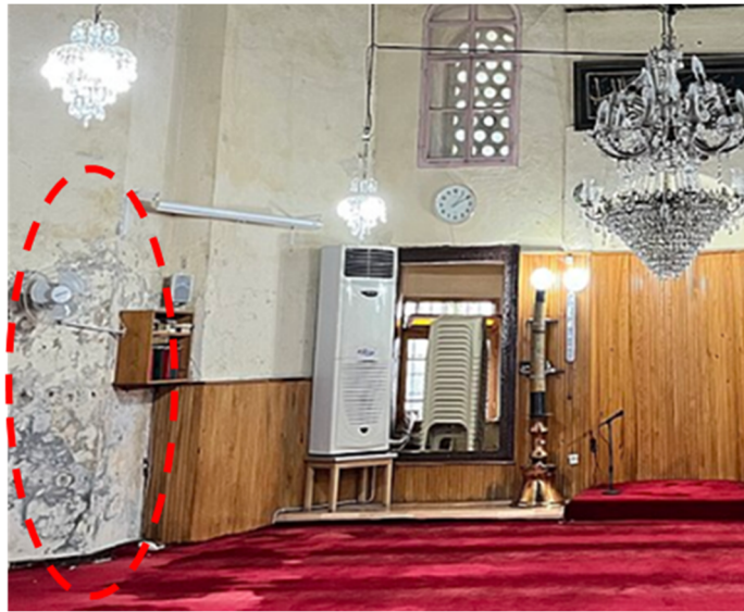
Figure 7. Persistent issue of dampness and humidity within the mosque.
