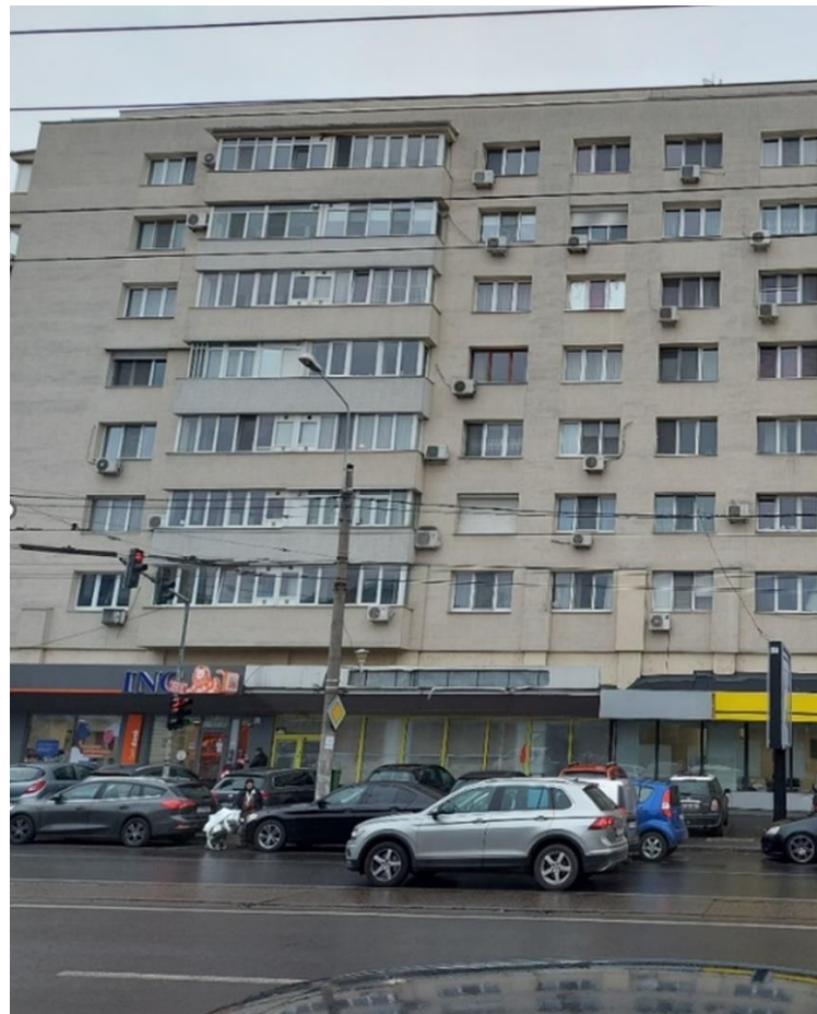
Figure 2. A soft-story structure that was heavily damaged during the Vrancea 1977 earthquake and that was recently thermally retrofitted without additional structural interventions.
