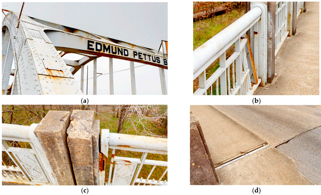
Figure 4. Places of the bridge needing maintenance and repairs. (a) Corrosion and paint maintenance needed along Span-2. (b) Damaged railing plate and baluster on Span-8. (c) Chipped and damaged cast-in-place concrete stanchion and broken baluster on Span-7. (d) Damaged expansion joint and missing cover plate near the north approach ramp.
