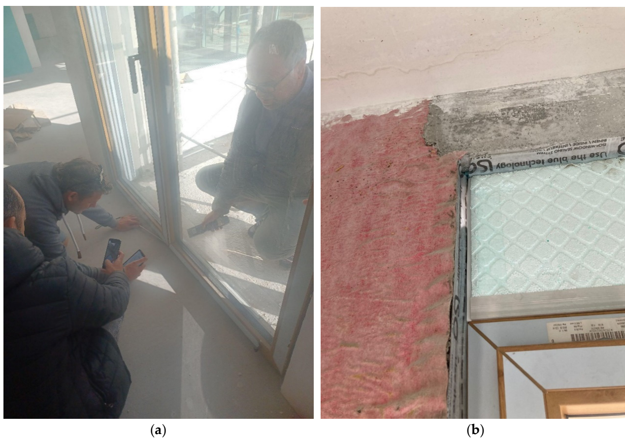
Figure 5. (a) Detection of air infiltration after phase P1; (b) Details of sealing using adhesive tape.
