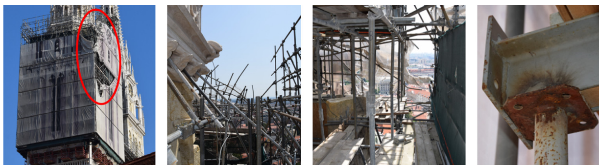
Figure 11. Damage on the old scaffolding structure on the south tower of Zagreb Cathedral [36].
