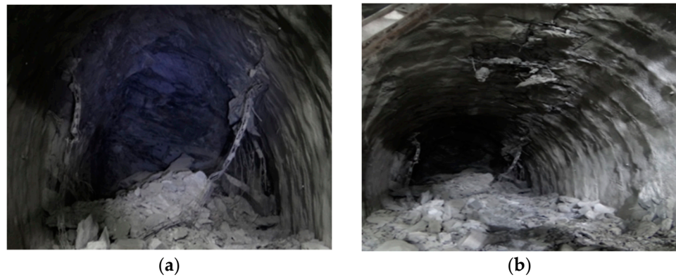
Figure 3. Left line of Ping'an Tunnel strong rockburst outbreak site: (a) Strong rockburst (D8K160+990). (b) Strong rockburst (D8K171+938).
