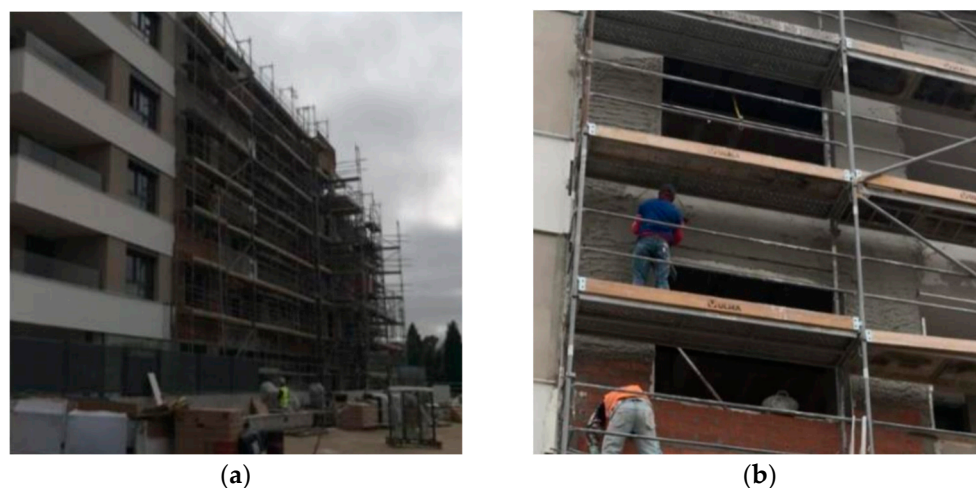
Figure 5. Work unit: (a) location of the work area within the construction site; (b) status of the execution area of the work unit.
