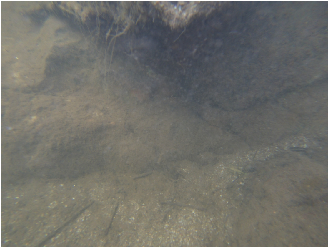
Figure 9. Underwater drone image of the junction between the foundation and the riverbed (photo by the author). This was the only singular point discovered during the underwater inspection, but it was not dangerous.
