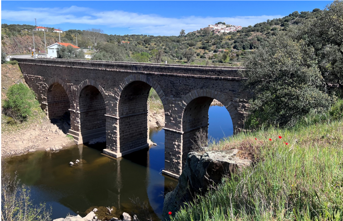
Figure 4. General view of the southern (downstream) side of the Segura Bridge, showing that it is a Roman masonry bridge with five arches, the central one being the largest (photo by the author).
