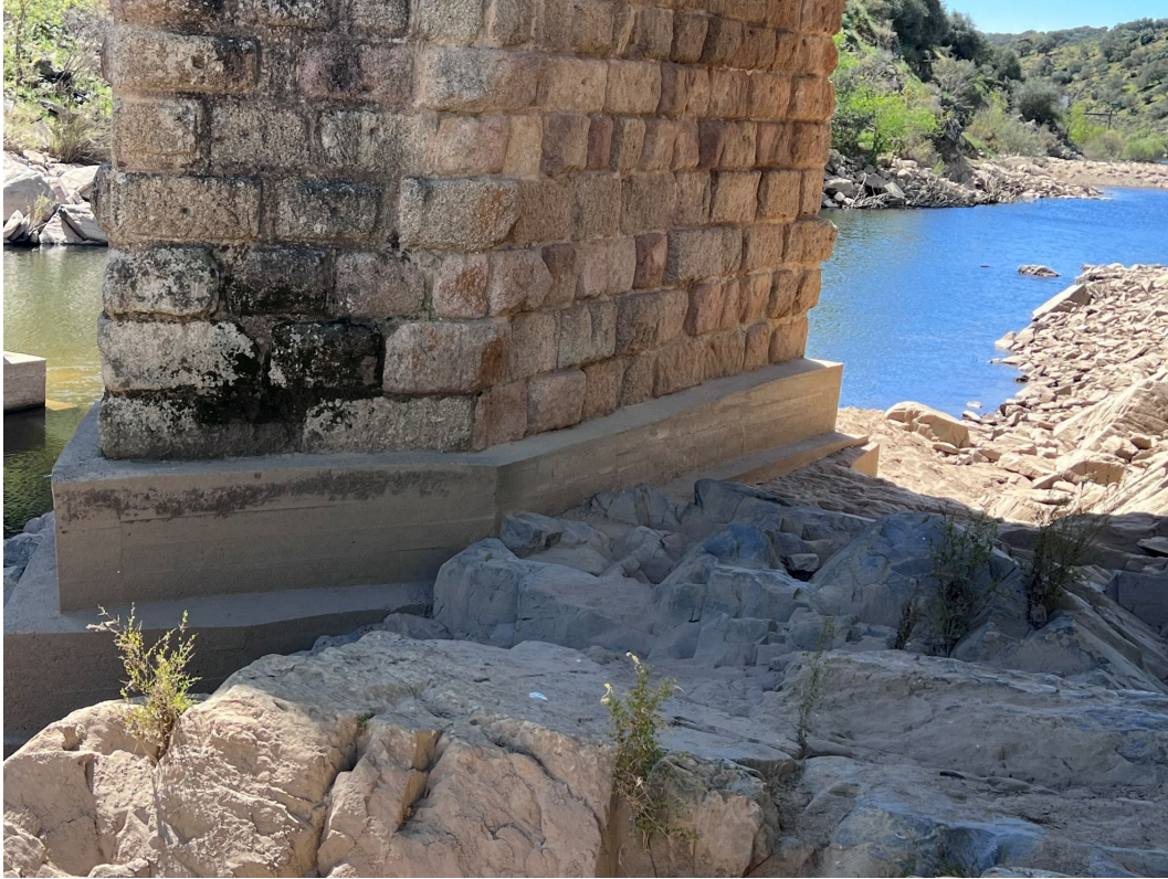
Figure 6. First pier, starting from the Portuguese side, showing the concrete casing and supporting rock (photo by the author).
