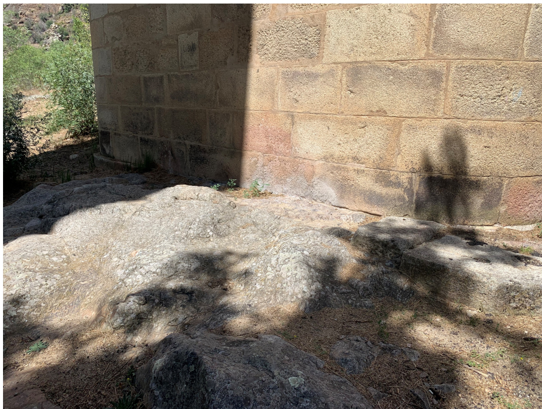
Figure 12. View of the first pier of the bridge, counting from the northern abutment (Zamora side), showing its support (photo by the author). This photo served to give an idea of the foundation of the bridge elements, as not all of them were visible.
