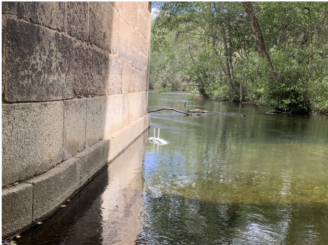
Figure 11. Underwater drone approaching one of the central piers of the San Lorenzo Bridge from downstream to allow observation of the submerged elements (photo by the author).
