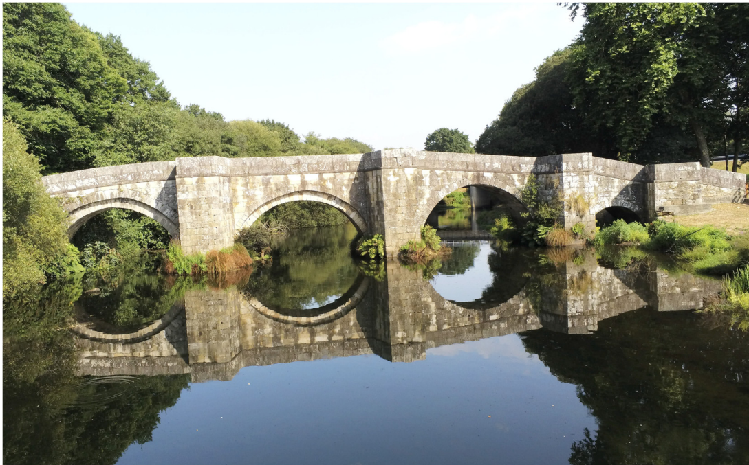
Figure 16. General view of the downstream elevation of the Brandomil Bridge, in an image captured by a quadcopter drone (photo by the author).
