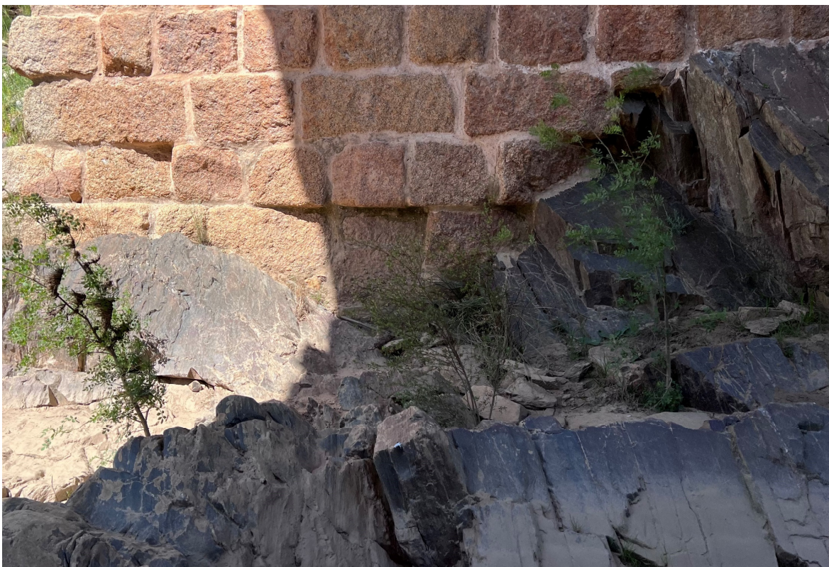
Figure 5. Close-up of the abutment on the Portuguese side, showing the arrangement of its first rows on the rocky material (photo by the author). This photo serves to give an idea about the foundation of the bridge elements because not all of them were visible.
