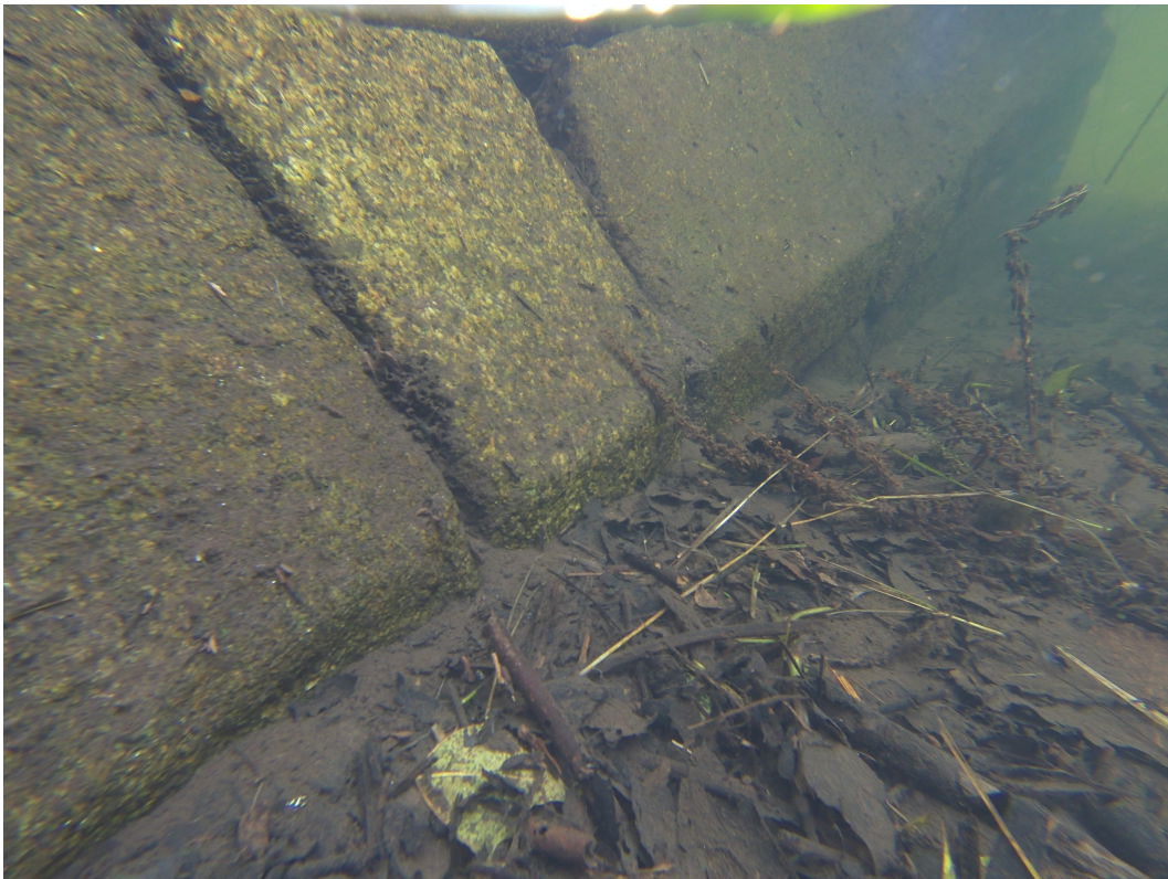
Figure 18. Underwater drone image of a fragment of the base of one of the central piers of the Brandomil Bridge (photo by the author).
