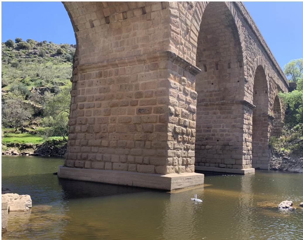
Figure 7. Underwater drone approaching one of the central piers of the Segura Bridge from downstream/the south (photo by the author). At that point, the drone made it possible to observe the submerged concrete lining and supporting rock.
