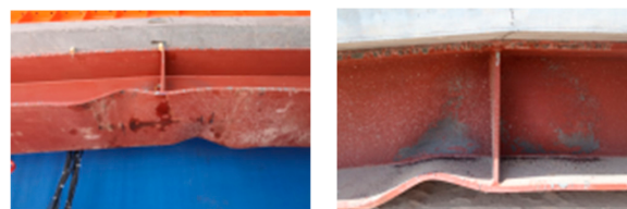
(a) Buckling of the lower flange of the steel beam
