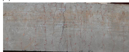
(c) Cracks on the surface of C50 concrete slab
