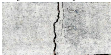
(b) Cracks on the surface of CA-RPC slab
