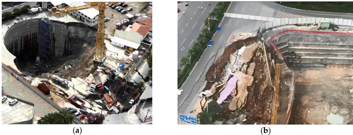
Figure 1. Subway pit collapse with extensive damage: (a) Singapore MRT foundation pit; (b) Nanning Greenland deep foundation pit.
