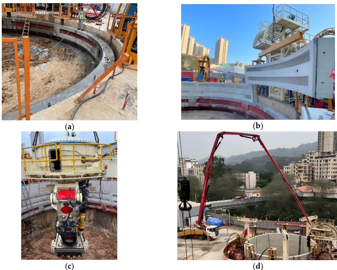
Figure 4. Mechanical shaft sinking method construction process: (a) cutting edge positioning; (b) 0-ring segment splicing; (c) shaft excavation machine installation; (d) underwater grouting.
