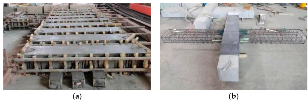
Figure 7. Manufacturing of the column: (a) pouring of the concrete; (b) connection of II-shaped steel and the longitudinal bar of the beam.
