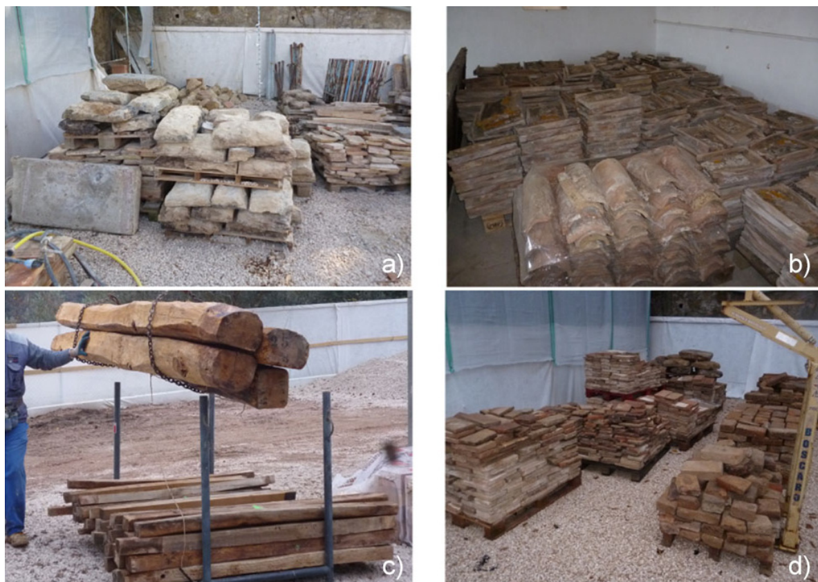
Figure 5. Existing materials found in the historic building and reused during the refurbishment: (a) recycled stones; (b) recovered roof tiles; (c) rescued wooden beams; and (d) recycled original bricks.
