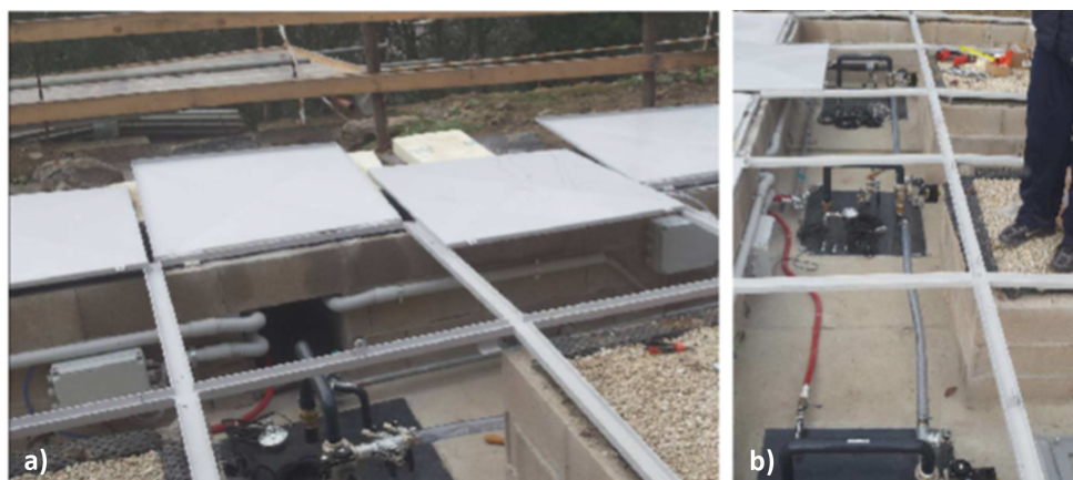
Figure 13. Front (a) and side (b) view of the bio-gas plant.
