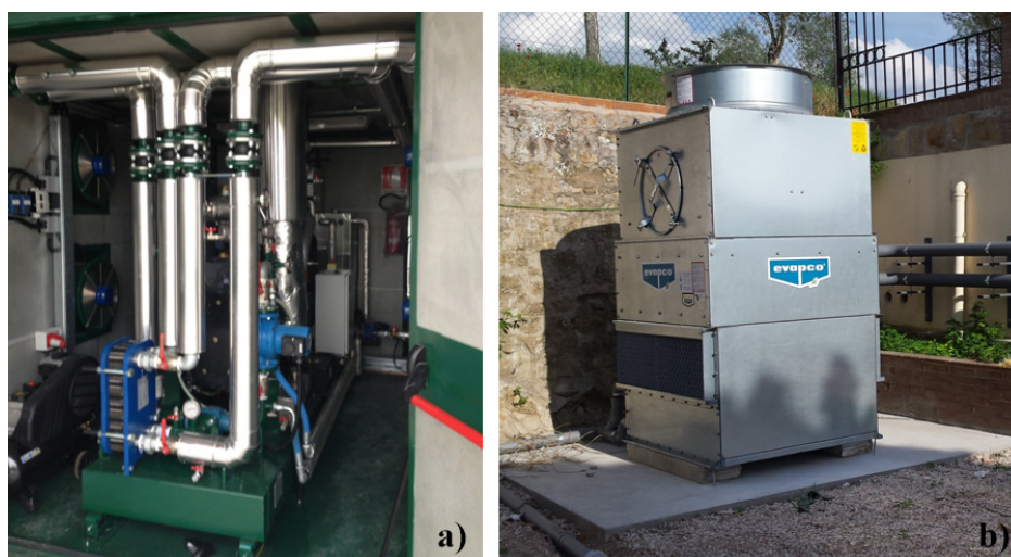
Figure 12. Cogeneration vegetable oil plant (a) and cooling tower (b).
