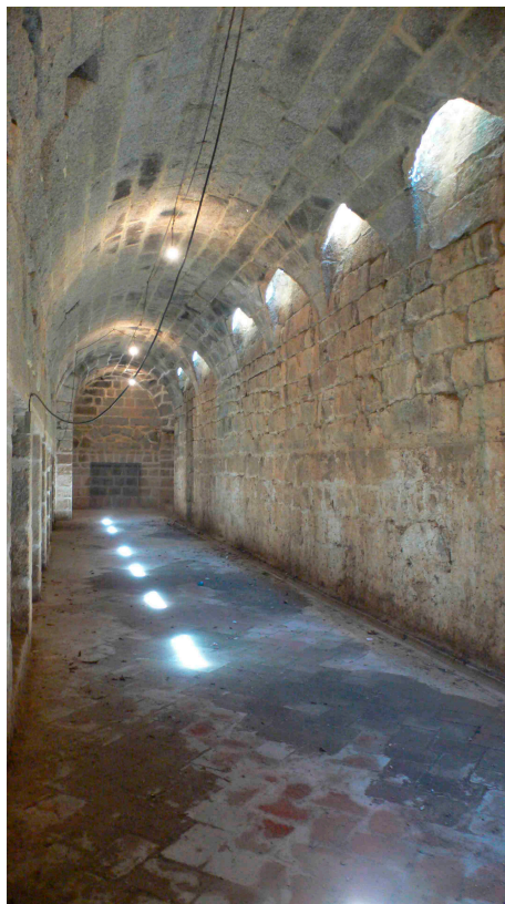
Figure 19. The lower cellar of the Galería from the south. Photograph by the authors.
