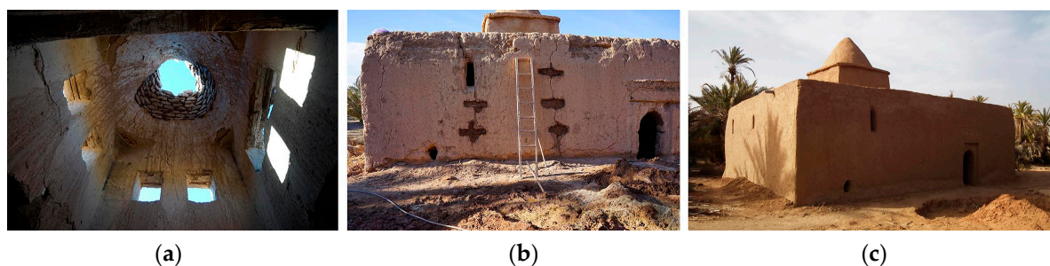
Figure 11. (a) Reconstruction works of the vault using adobe; (b) Sewing the wall with wooden keys; (c) Current status after restoration.
