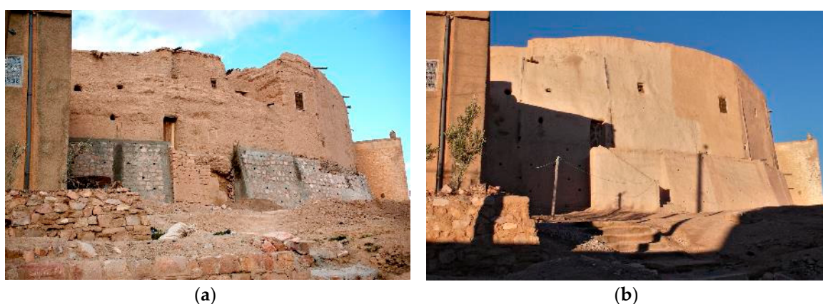
Figure 3. Restoration of the Tachaouite Ksar. (a) During the restoration work; (b) Final result.
