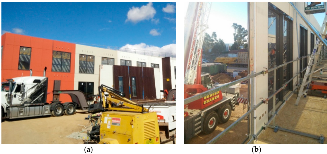
Figure 16. Implementation with panelised form of prefabricated construction: (a) Commercial office building using the gasket seals; (b) EPDM gasket seal positions on the wall towards the outside face.
