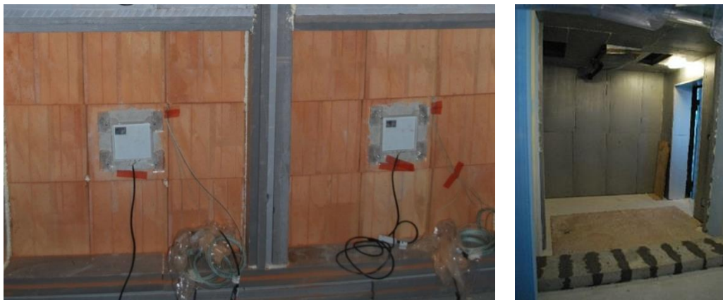
Figure 2. View of the partitions made of modified ceramic elements and the interior of the cold chamber—the preparatory stage.
