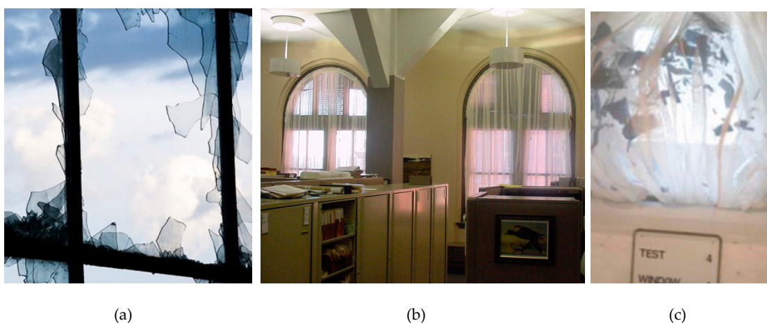
Figure 14. Glass windows and facades under shock: (a) example of severe damage of un-protected window and (b,c) enhanced performance in presence of textile curtain nets.
