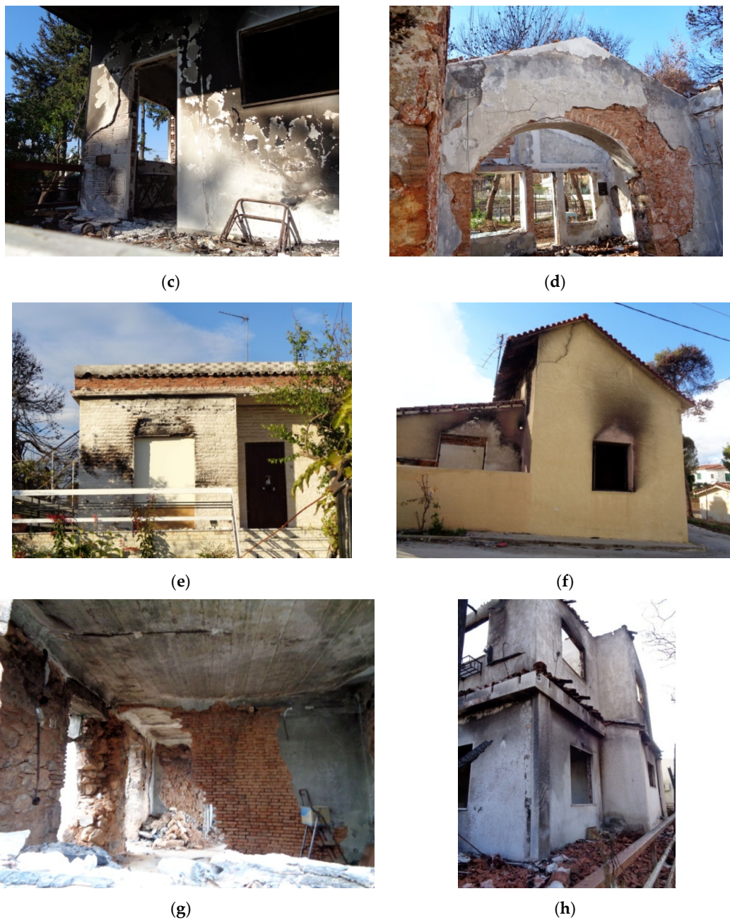
Figure 6. Photographs of damage in masonry buildings after the wildfire in Mati: (a,b) discoloration of exposed surfaces; (c–f) cracking of walls; (g) extensive damage; (h) destroyed wooden roof.
