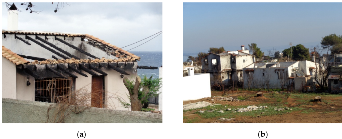
Figure 7. (a,b) Photographs presenting damage that occurred in wooden roofs after the wildfire in Mati.
