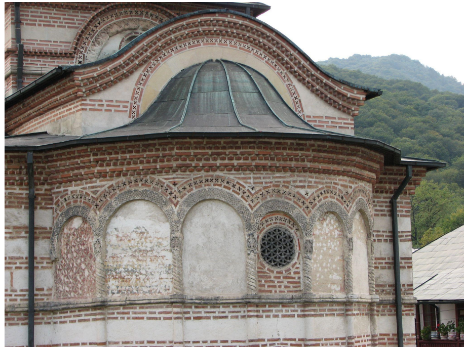
Figure 15. Exterior view of the upper portion of the church, showing the plastered and painted surfaces under the arches, Cozia Monastery, Wallachia, modern-day Romania (source: Elisabeta Negrău).
