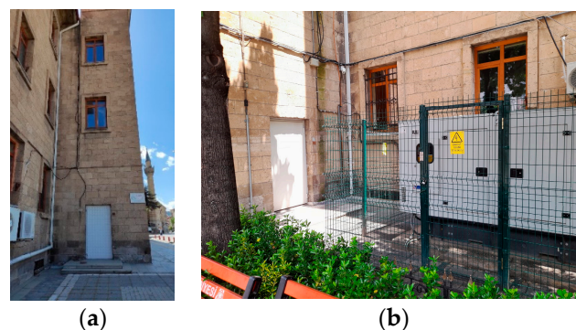
Figure 11. Fire escape and entry: (a); exit doors: (b). Photo by Nurcihan Akdağ 10 June 2023.
