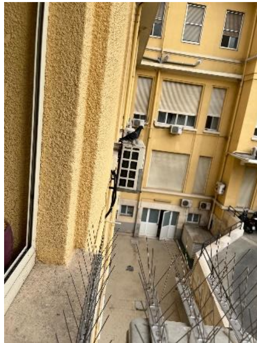
Figure 2. Several external air conditioning units installed under the windows of public offices.
