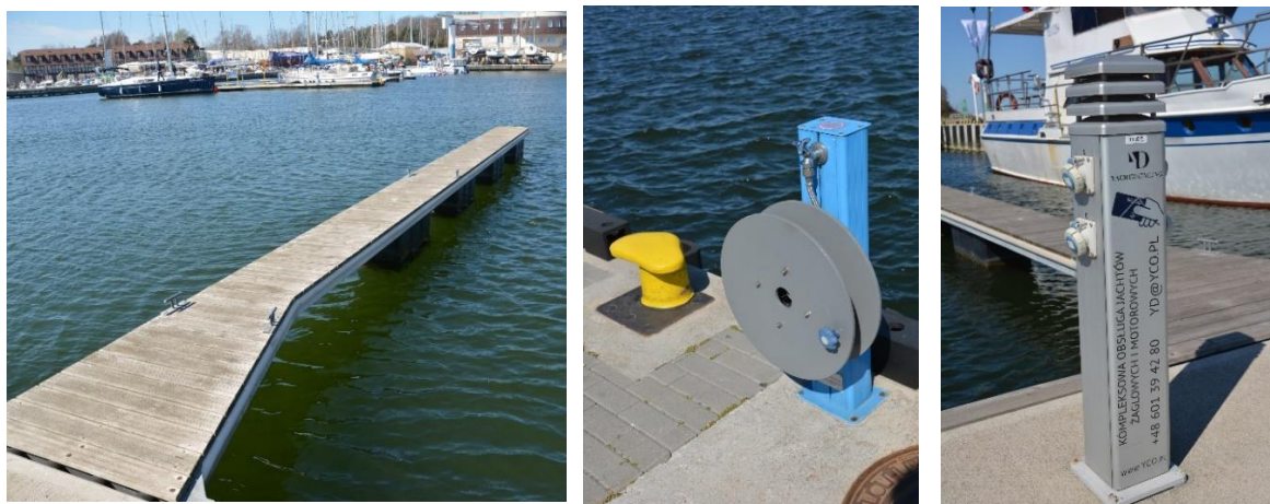
Figure 6. A platform and components of infrastructure: a hydrant and an electrical container.
