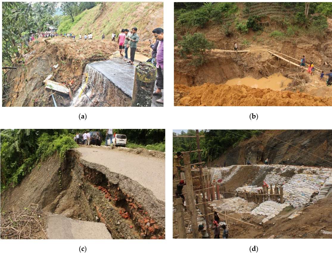
Figure 2. (a) Part of the Rangamati-Chattogram road collapsed at Manikchhari; (b) people had built a temporary solution after the local road had been damaged near the Rangamati-Khagrachari road; (c) heavily damaged Rangamati-Manikchhari road; (d) temporary measures were taken on the Rangamati District road to reestablish the road network.
