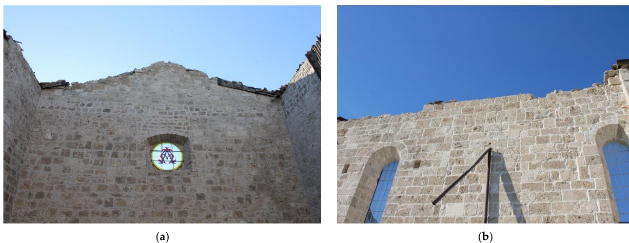
Figure 25. Limited damages and loss of usability in the Abbey in Montesanto (C25): (a) absence of damage in the façade and roof collapse; (b) absence of damage in the lateral wall.
