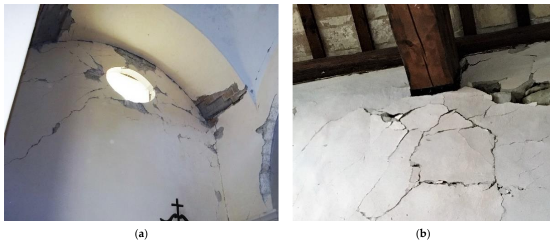
Figure 20. Other mechanisms activated in the wall: (a) shear mechanism in the lateral walls in St. Giovenale church in Roccasalli (C25); (b) roof covering mechanism in St. Elpidio church in Campli (C9).
