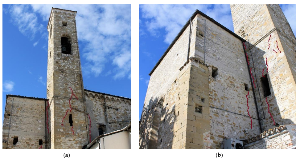
Figure 18. Damages on the stem of the belltower (a,b): the case of the St. Francis church in Campli (C23). The observed crack pattern has been highlighted in red.
