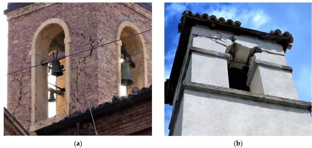
Figure 19. The structural component of the bell cell: (a) the case of St. Savino church in Gualdo (C36); (b) the case St. Maxim Oratory in Collalto, Amatrice (C8).
