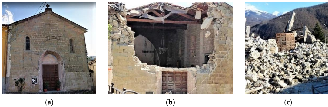
Figure 10. The St. Lawrence and St. Paul Church in Accumoli: (a) before the Central Italy earthquake; (b) after the 24 August strong motion; and (c) after the earthquake occurred on 30 October 2016.
