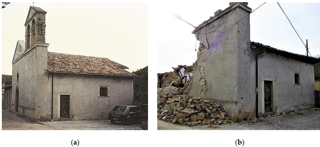
Figure 12. The St. Peter and Paul church in Macchia (Accumoli), before (a) and after (b) the earthquake occurred on 30 October 2016.
