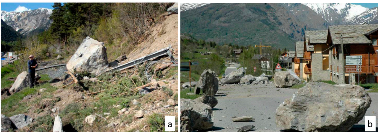
Figure 4. Some of the blocks that detached from the slope during the 2010 event and caused damage to the existing rockfall barriers (a) and the SP 216 road (b) [18].
