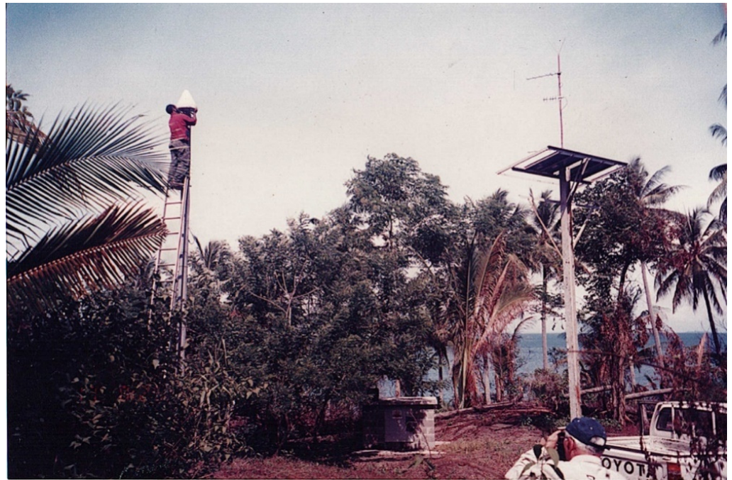
Figure 7. The Remote site at Vulcan (VIS) in 1999. A concrete bunker to house the receiver, telemetry, power, etc., is in the centre. Left, a choke-ring antenna is being placed on a 6 m pole (to avoid rapid tree growth). Right, a solar panel mast, with telemetry yagi antennas. The opportunity was taken to co-host seismometers in the bunkers. (Photo by author.).
