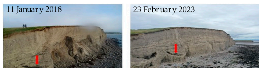
Figure 12. Removal of the prominent talus slope between 11 January 2018 and 23 February 2023. For reference, the red arrows mark the same feature (a deformed lens of glaciofluvial material) in both photographs.
