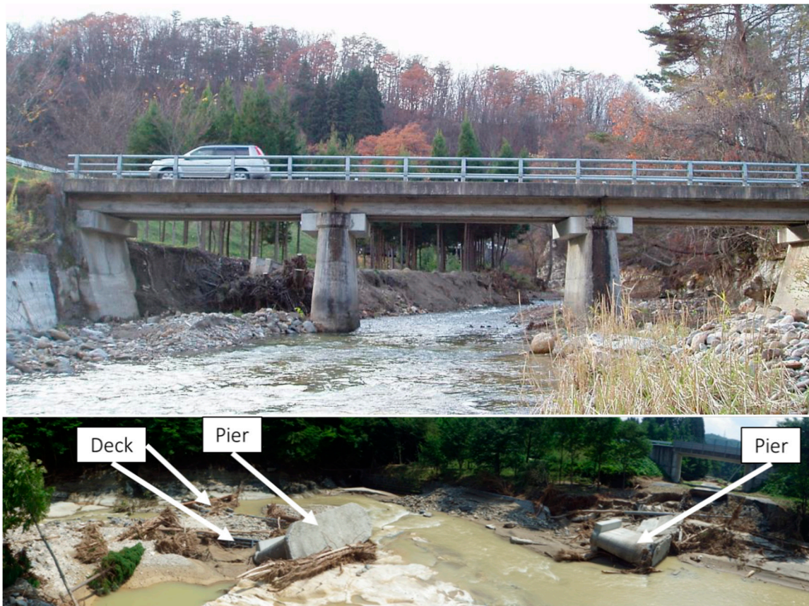
Figure 3. Yabitsu bridge before flood ( upper ) and after ( lower ).
