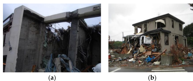
Figure 2. Evidence of debris effects on buildings, from the 2011 Japan Tsunami. (a) Likely large debris impact on the top floor of an overturned Reinforced Concrete-framed building; (b) Openings dammed by debris. (Photos: [4]).
