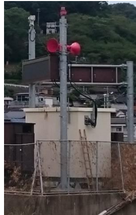
Figure 5. Siren and loudspeaker of the dam operator.
