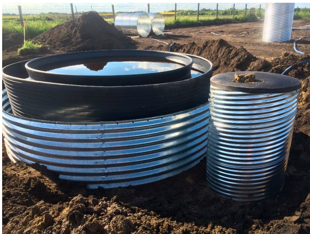
Figure 1. Mesocosm protected by steel tunnel liner and overflow tank housed within a culvert, visible during construction in 2016.
