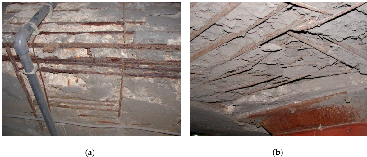
Figure 3. Examples of steel damage in one of the structure C: (a) corrosion of steel rebars with concrete damage, (b) locally interrupted reinforcement.
