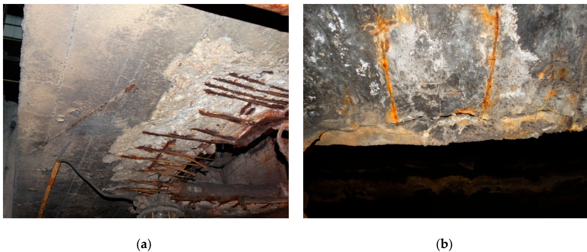
Figure 4. Examples of corrosive damage in A facility: (a) concrete and steel corrosion, (b) traces of completely corroded stirrups.
