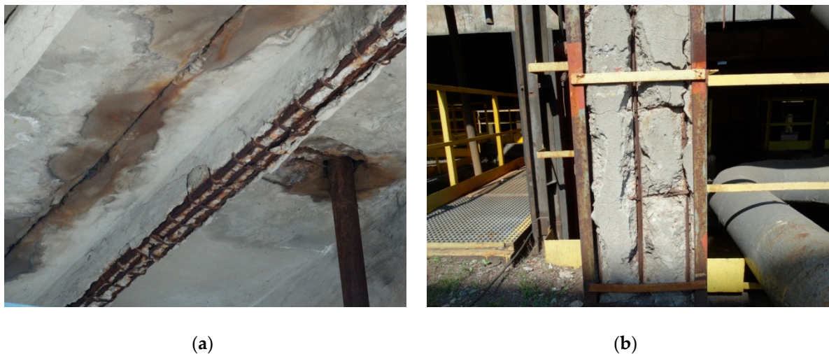
Figure 6. The very bad condition of structural elements: (a) swelling steel rebars caused damage of the concrete cover, (b) damaged steel strengthening and concrete of columns.
