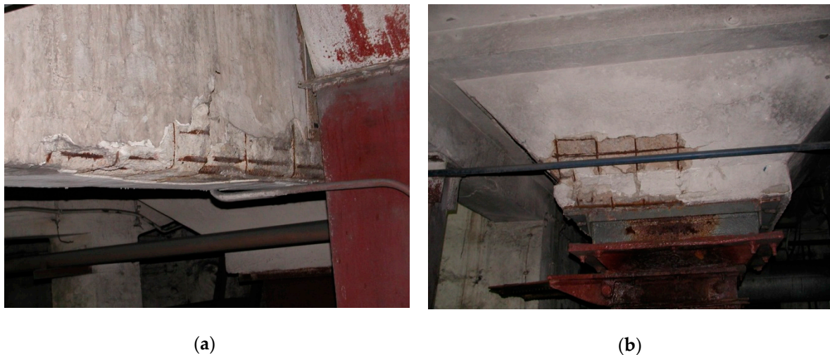
Figure 2. Examples of corrosive damage: (a,b) corrosion of steel rebars in defected concrete cover.
