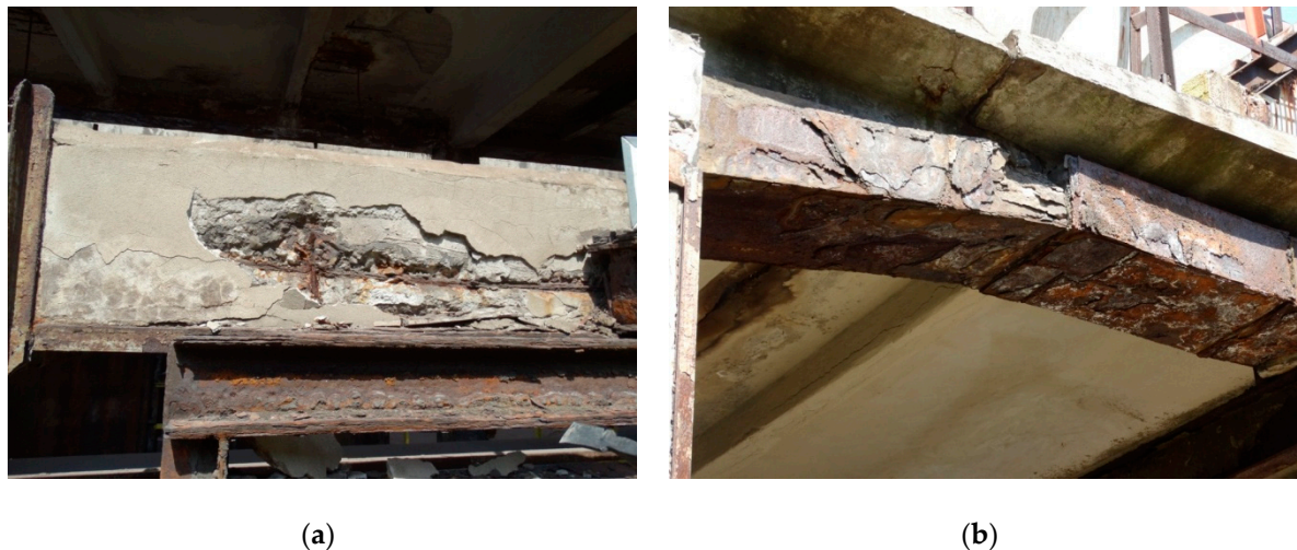
Figure 5. Damage of varying intensity: (a) damage of concrete and steel corrosion of rebars and profiles, (b) strong corrosion of steel elements used as the strengthening of concrete beams.
