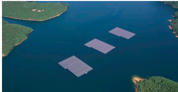
Figure 2. Three MW floating PV systems on the reservoir of Chungju Dam, Korea (source: K-water).
