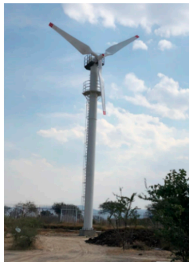
Figure 4. Three-blade wind turbine installed on Universidad Autónoma de Querétaro (UAQ).
