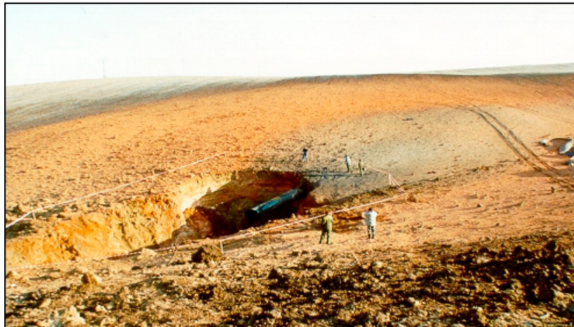
Figure 8. Gas pipeline accident due to the additional bending of a pipeline system laid on a slope with insufficient amounts of compacted subsoil.
